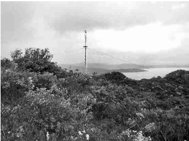
Going up... Construction of the wind monitoring mast began in August last year, behind the lime quarry above Ocean Beach. Data since collected indicate that the proposed windfarm site has exceptional wind capabilities.
